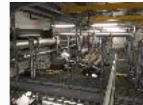
Alderley Park Energy centre upper level
