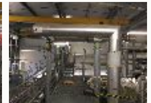
Alderley Park Energy centre ground level.
